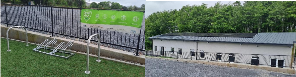
Coolkenno Sports, bicycle parking and solar PV installation
